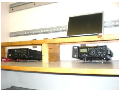
Donated Yaesu FT 897 (160 through 10 plus 6 meters 2 meters & 70 CM) & ICOM 7200 (160 through 10 plus 6 meters) installed in Communications Vehicle and awaiting antennas
